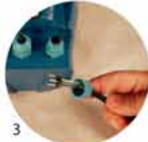
3 a) you must use a cable with a round cross-section b) you must use a cable with 3 conductors (twin and earth)
